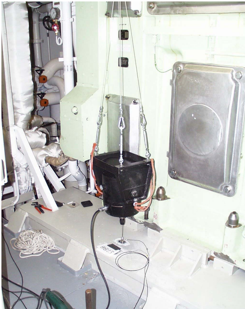
Figure 5. Installation of shaker, engine bed with mounted engine in the ship (excitation point BB13).
