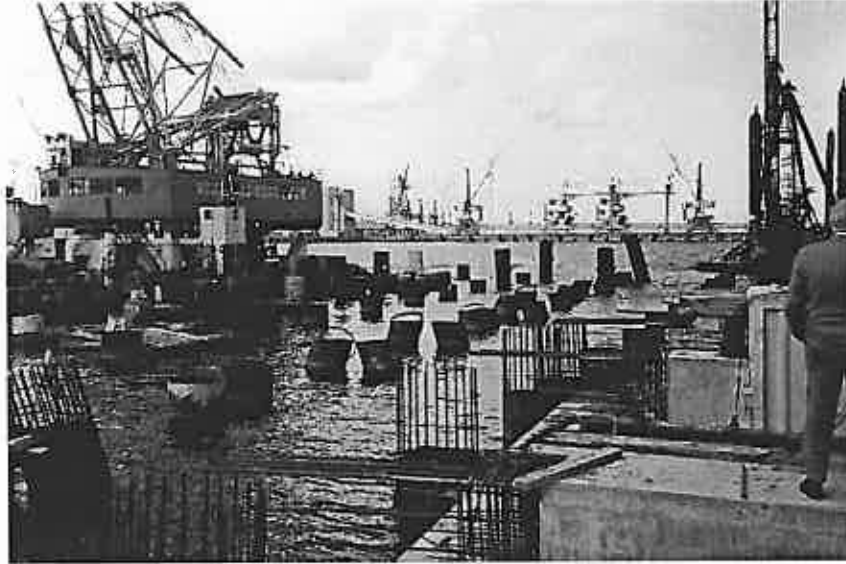
Figure 13. New pier for the RoRo terminal of the Port of Muuga under construction, summer 2000.
