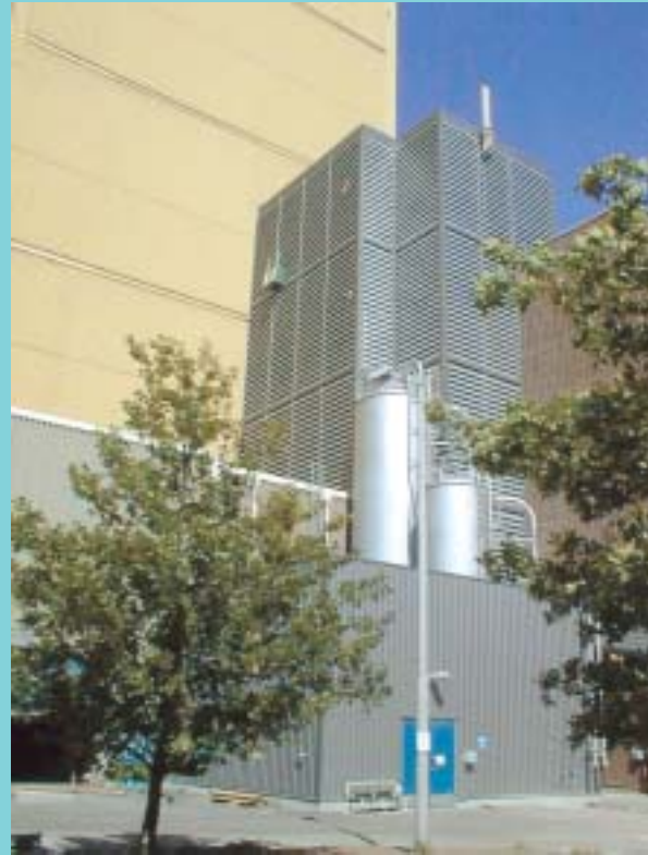
The Lahti CFB gasifier which is connected into 350 MW pulverised coal fired boiler has been in operation since 1998. Lahti Energia.
