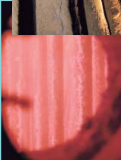
Deposits on superheater tubes. VTT Processes.
