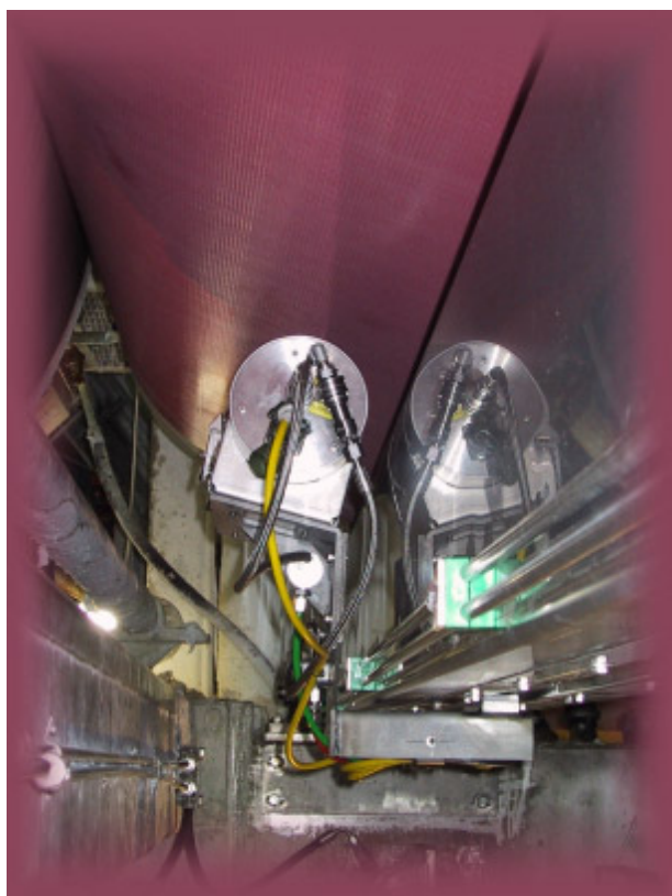
Figure 3. Moisture analyser installed on a paper machine. Photo by Metso Paper Inc.
