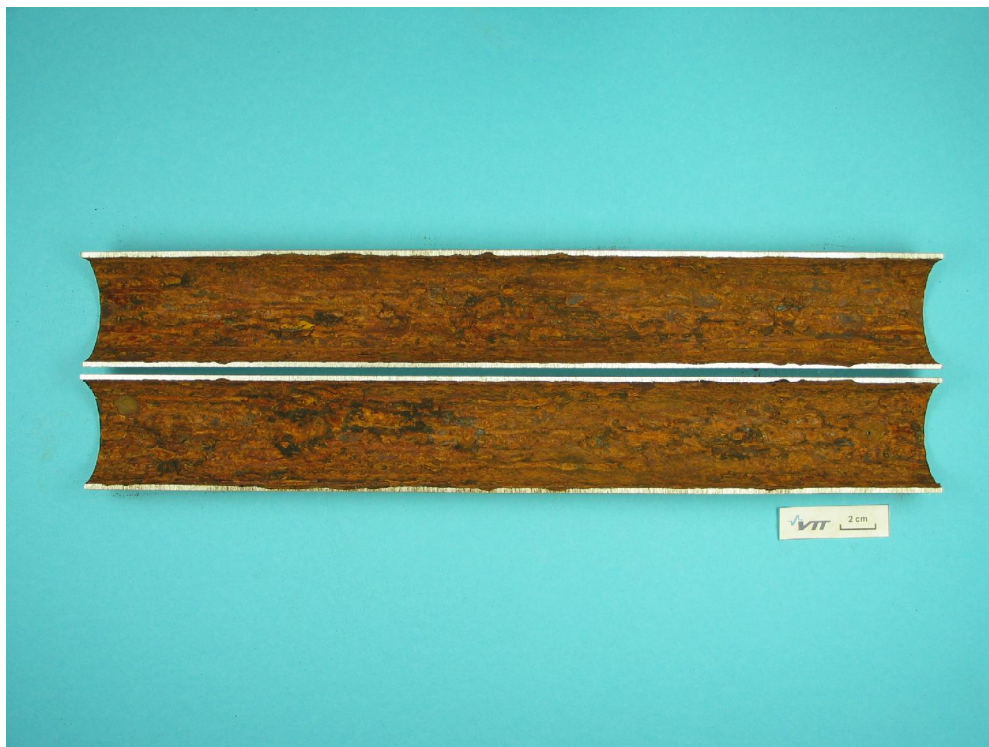
Figure 1. A piece of carbon steel pipe taken from a fire extinguishing system of a stainless steel factory after 20 years of use.
