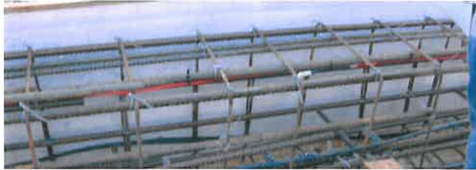
Figure 4.1.3. A 40 m long fibre optic sensor (VK3E2) and a Sahlen sensor were installed close to the same reinforcement.
