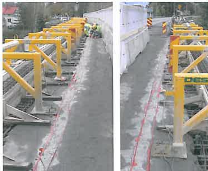
Figure 4.1.3. Fibre optic temperature sensors (VK4 E1 and VK4 E2) installed to the old part of the bridge deck.
