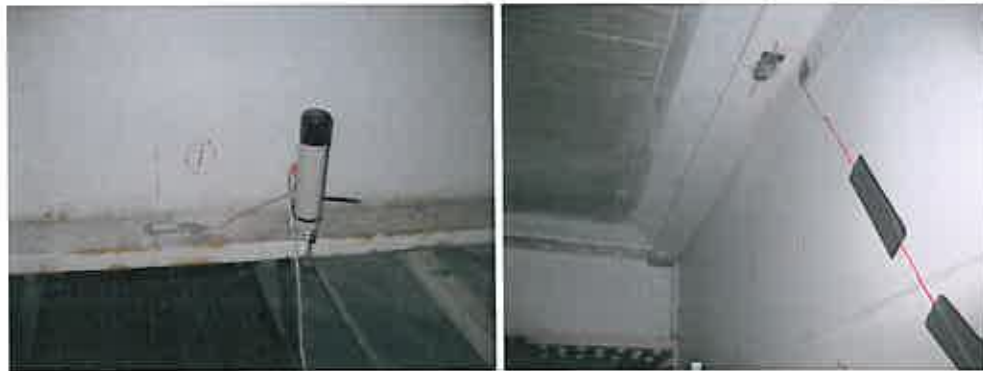
Figure 5.1.3. In the Hännilänsalmi bridge the strain gages have been fixed on the flanges of I-shaped beams.
