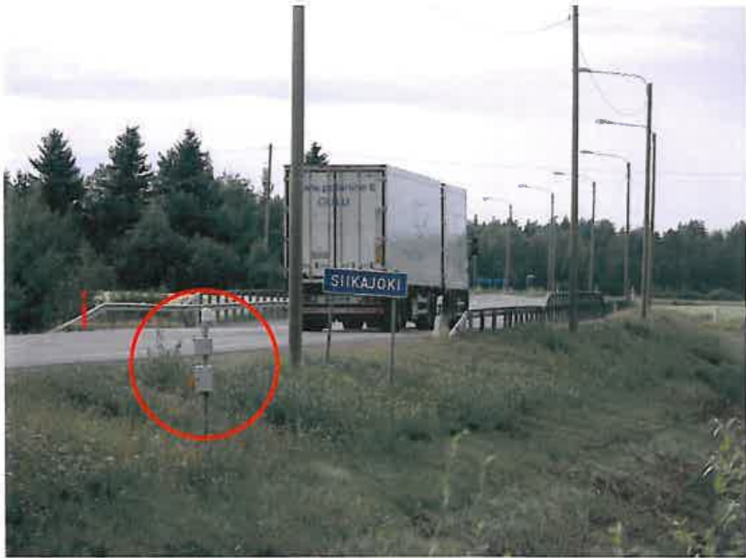
Figure 6.3.2. WSP's prototype of automation based monitoring system (circled) on the Jylhäranta Bridge.
