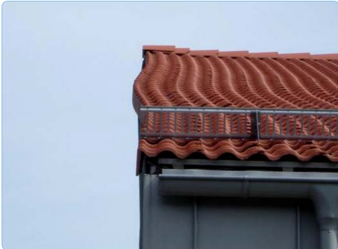
Figure 1. Buckling of the roof structures due to insufficient bracing [1].
