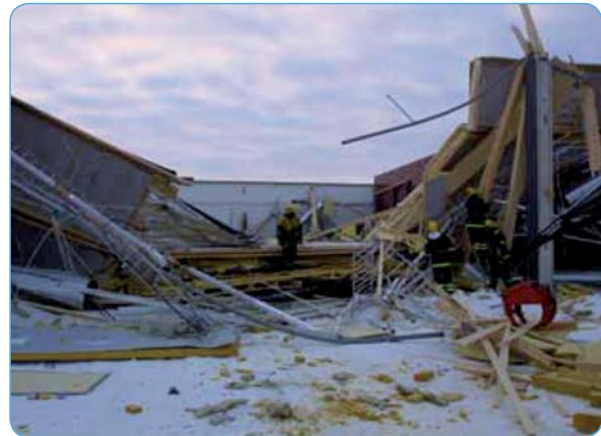
Figure 2. Collapse of the roof of a fair centre [1]
