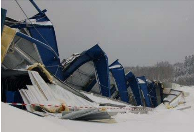
Figure 1. Typical LTB failure of a portal frame structure [2]
