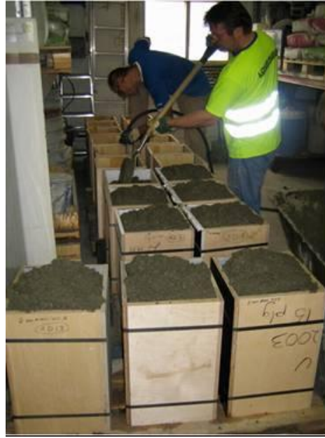
Figure 13. Casting of field specimen for field chloride penetration studies at Rudus Oy.
