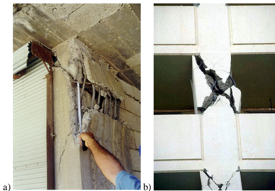
Figure 6. Shear failure of columns due to (a) inadequate spacing of shear reinforcement, (b) short-column effect
