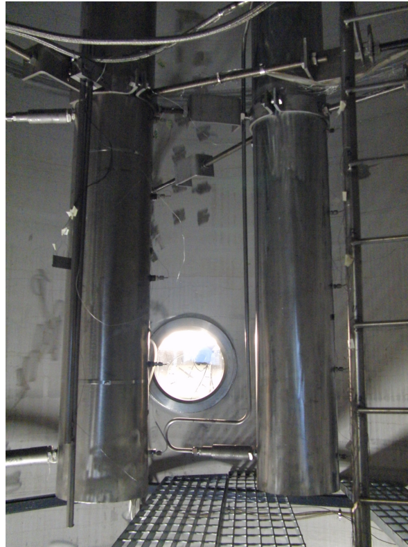
Figure 1. Parallel blowdown pipes in the PPOOLEX facility.
