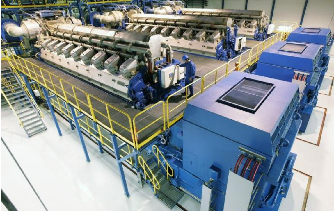
Figure 1. Wärtsilä 18V50 gensets with ABB generators in a power plant configuration [Wärtsilä Power Plants].
