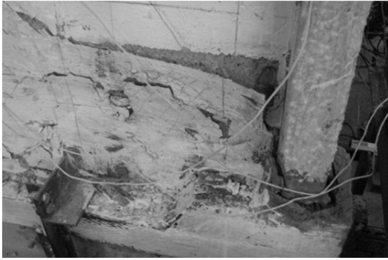
Figure 15. Shear strips debonding
