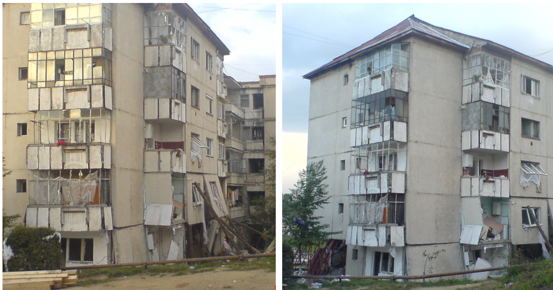
Figure 5. Ground floor external walls destroyed in a gas explosion in 2007, Zalău, Romania (Photos by Andrea Soós).
