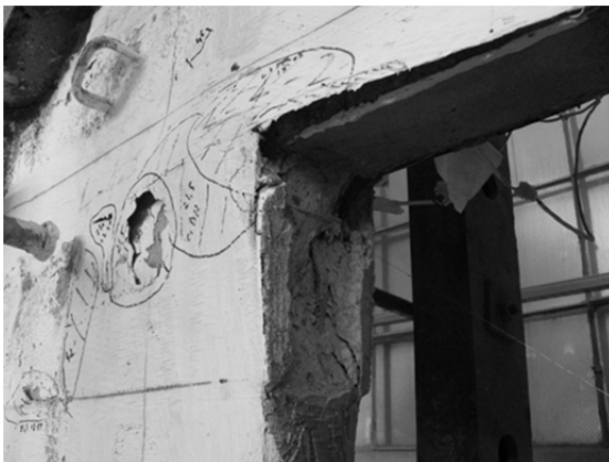
Figure 25. Flexural strip swelling, confinement strip rupture and concrete crush [3]
