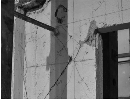
Figure 27. Flexural strip swelling, confinement strip rupture and concrete crush
