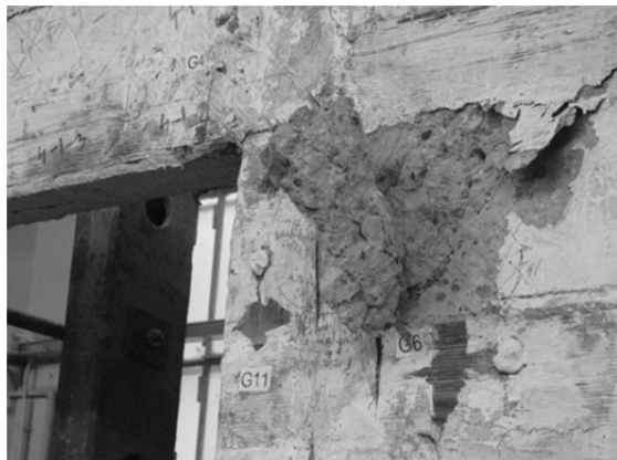
Figure 14. Confinement strips rupture
