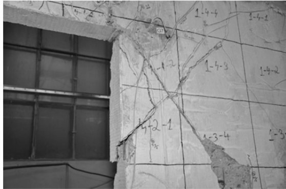
Figure 10. Concrete crushing of door corner
