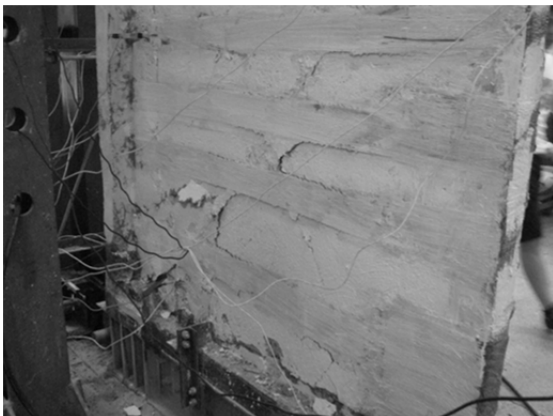
Figure 13. Shear strips debonding
