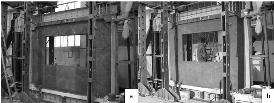
Figure 7. Application of a) glass fiber grid and b) second layer of mortar for the PRCWP (10-L1/L3-T/R) [10]
