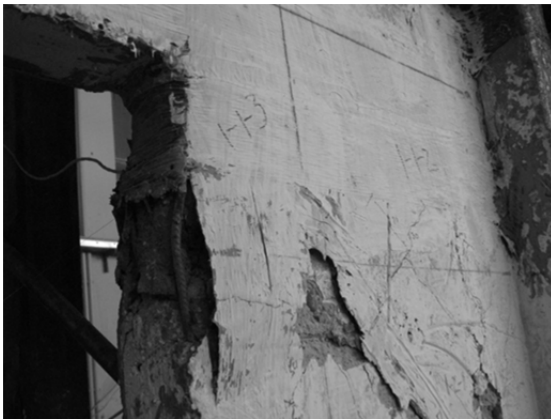
Figure 23. Flexural strip swelling and concrete crush
