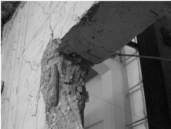
Figure 17. Upper left door corner crushing
