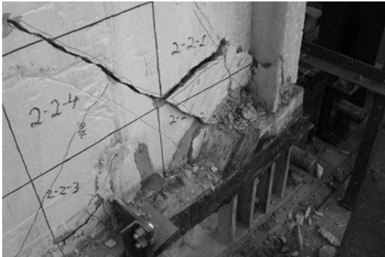
Figure 11. Panel bottom right corner crushing
