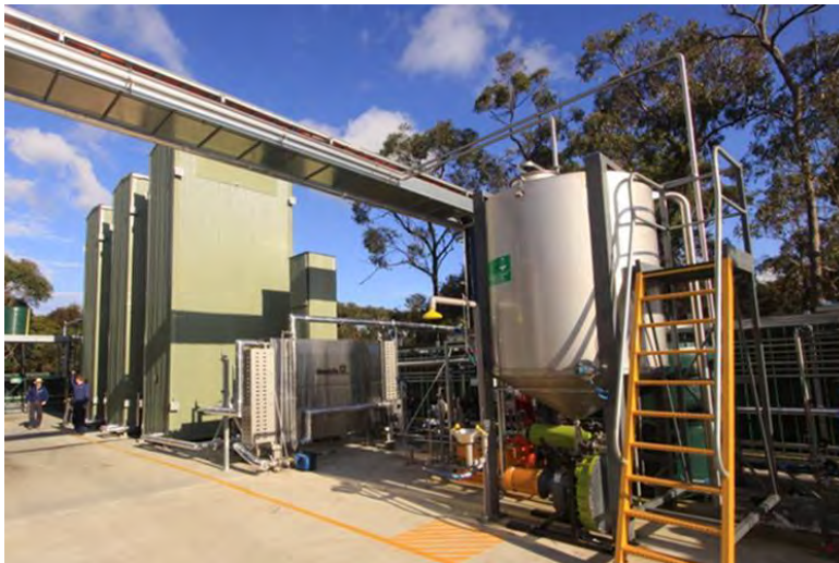
Figure 15. Licella commercial demonstration plant ( http://www.licella.com.au/about-us/commercial-demonstration-plant.html ).
