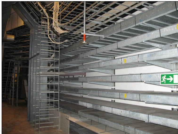
Figure A3. A photograph of part of the cable tray system. The eight lowest levels of cable trays (protected) contain IC-cables of sub-system B and the higher levels (unprotected) contain power cables of the same sub-system. Cable trays of sub-system D are located on the opposite side of the corridor (to the left in the picture).
