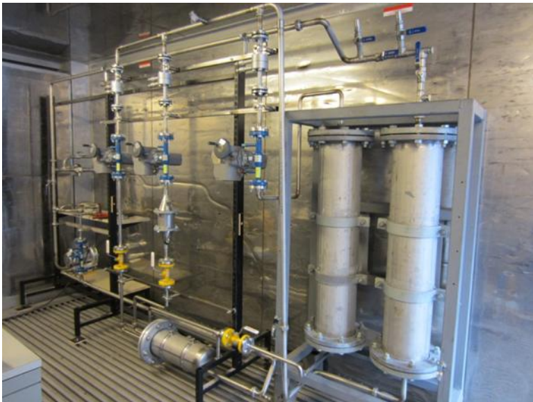
Picture 1. Picture of the siloxane removal test facility in project FCEP/WP4.2.2 - Minimum limit for biogas upgrading.
