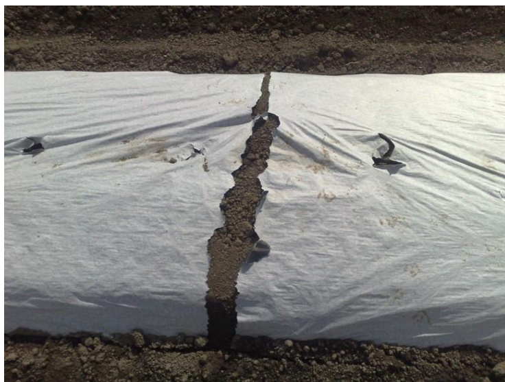
Figure 28. Tearing caused by shrinkage (UPM WEX WS)
