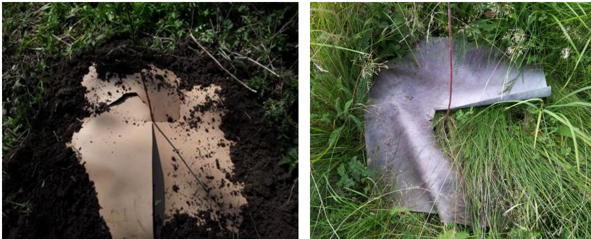
Figure 31. On the left: heat treated PGW board broken during installation. On the right: PGW board with the cutting line curled up and weeds growing through.
