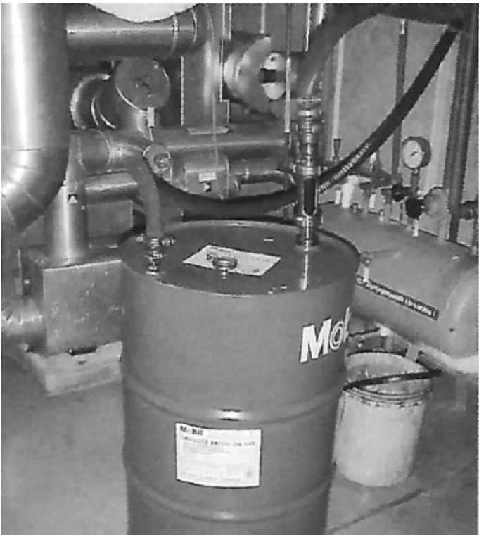
Figure 2. An oil recovery vat equipped with overfill prevention and a vent pipe leading outdoors.
