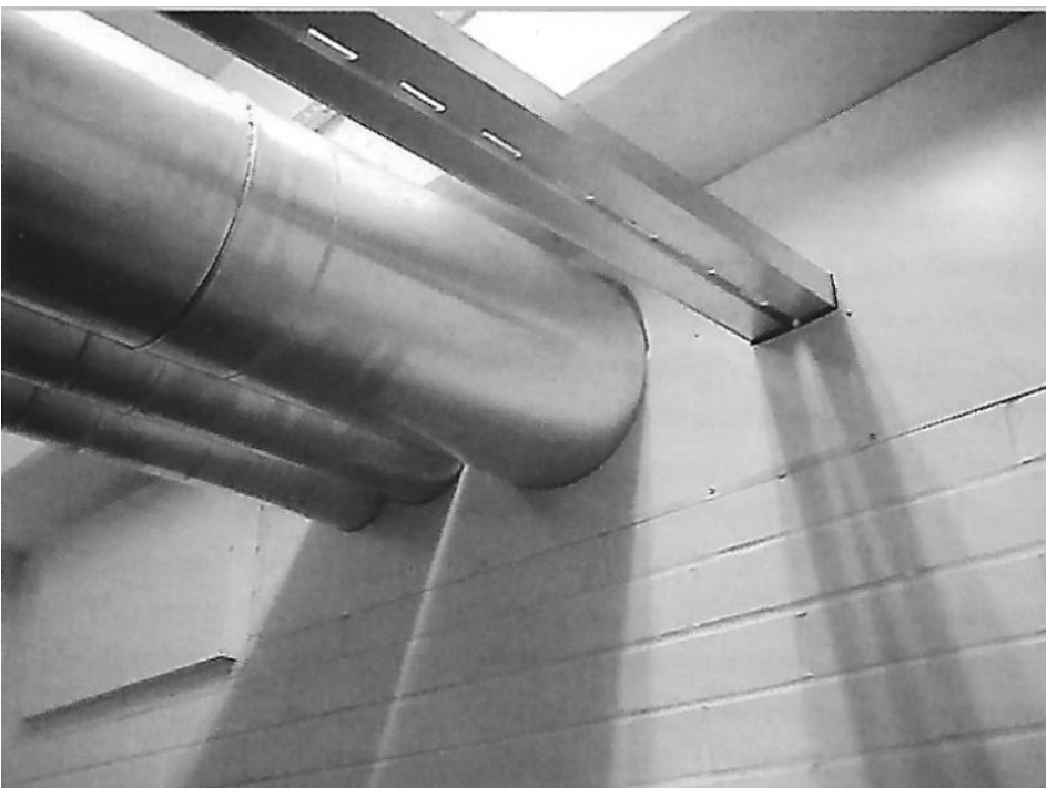
Figure 9. An example of lead-throughs of pipes. The pipes have been led through a large opening, allowing a continuous insulation. Besides, the opening has been sealed with mineral wool within the metal cladding.
