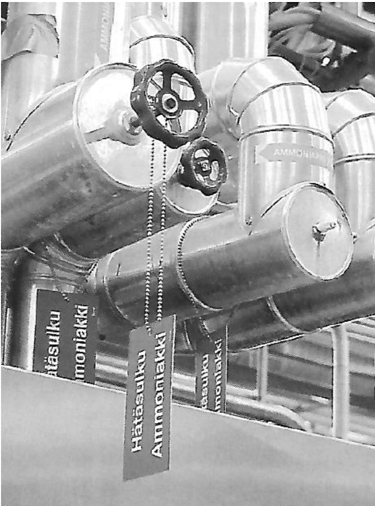
Figure 6. An example of the proper marking of valves and piping.
