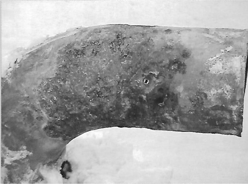
Figure 8. The hot gas pipe with the wet insulation removed.
