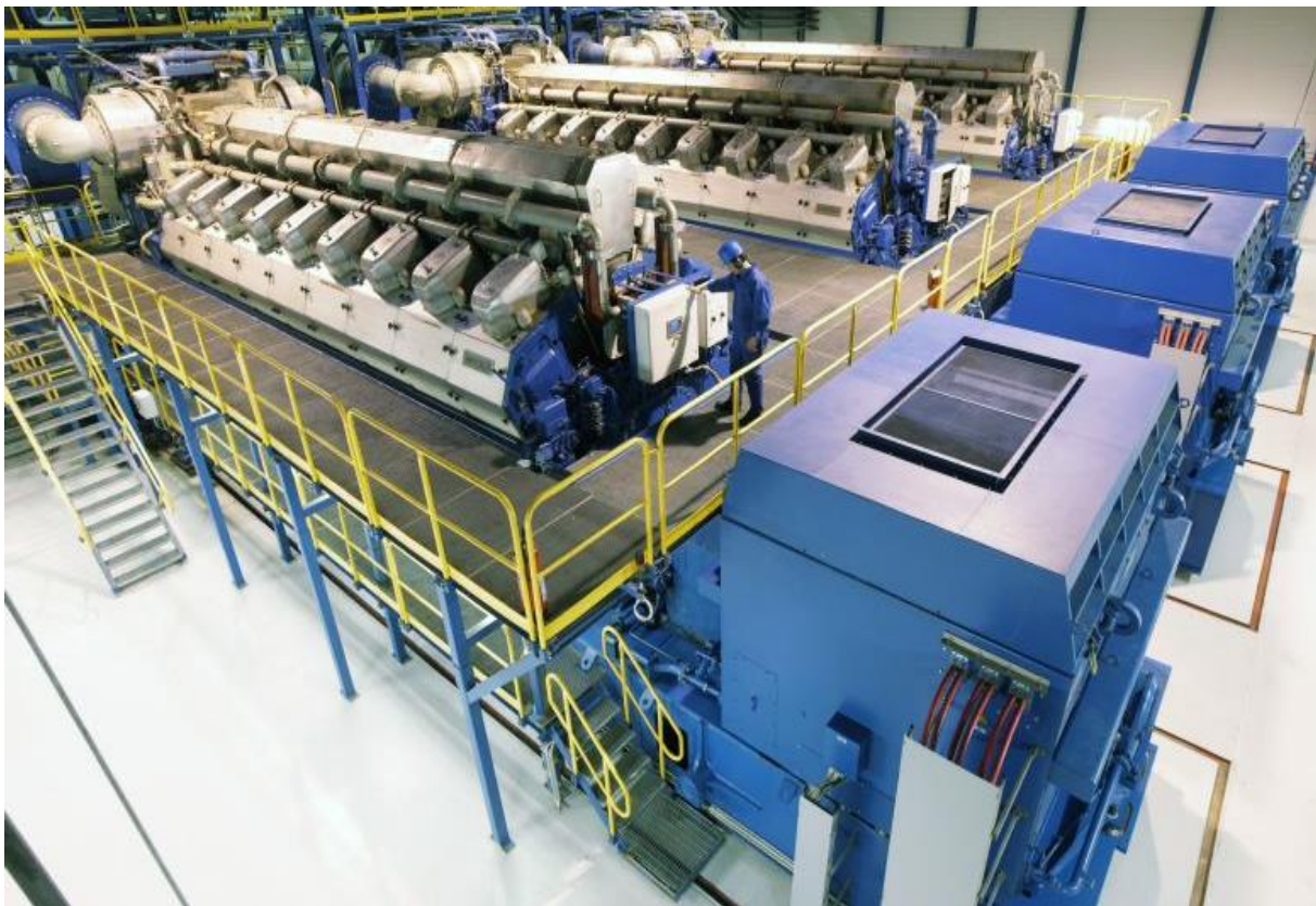
Figure 2. Diesel generating set (Wärtsilä Power Plants).
