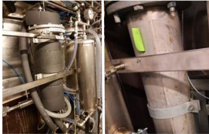
Figure 16: Left Figure 12a: Delay tank in the back a) Right Figure 12b) gas liquid separation tank.
