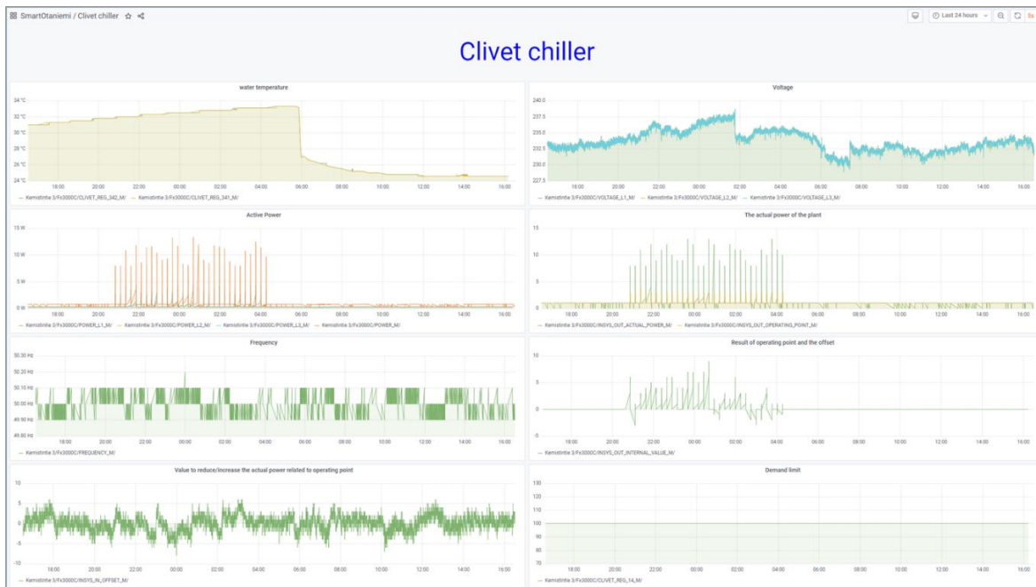
Figure 14. An example of a VTT research platform based chiller unit real-time monitoring dashboard (case Kemistintie 3 Clivet chiller unit via Fidelix FX-3000-C).
