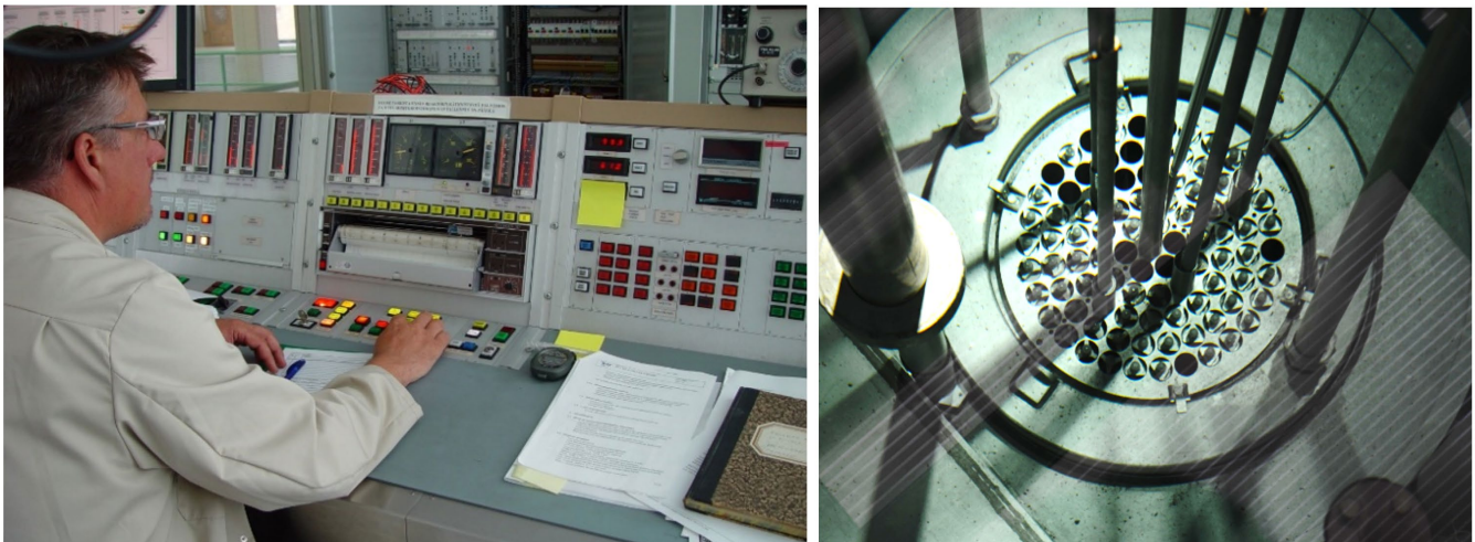
Figure 1. Reactor operator just about to shut down FiR 1 for the last time on 30 June 2015. At the end of the same year, the core was made permanently subcritical by removing a sufficient number of fuel elements.
