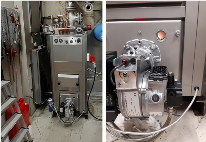
Figure 8 Ash generator based on an oil burner and a boiler installed in the eDyna test cell (left). Ash generator in operation (right).
