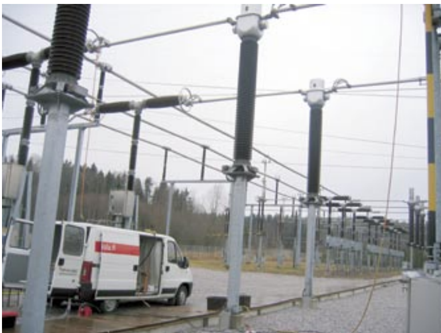
Figure E8. On-site calibration of a current transformer on the 400 kV grid. The current transformer under calibration is in the center of the picture. The orange cable hanging down from the high voltage line was used to feed the current, and the current generator together with the reference instrumentation were in the van.
