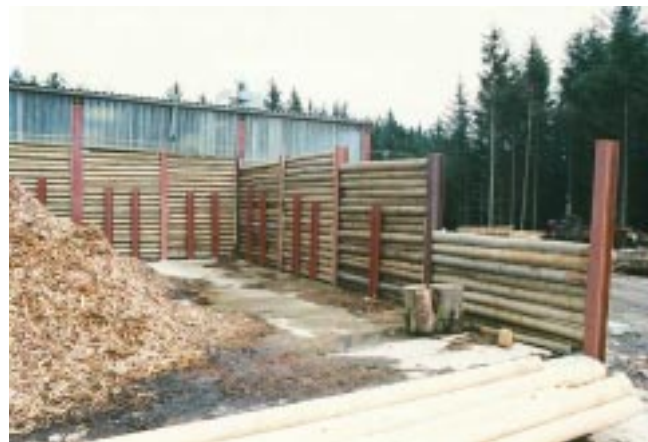
Figure 5.18. Storage bins combining round-poles and steel with added protection for machine loading operations.
