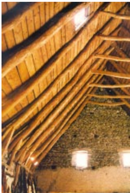
Figure 5.6. Round-pole rafters in a French barn now used as a craft shop.
