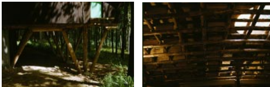
Figure 5.46. Support system and internal roof structure of scarf jointed poles for the Westminster Lodge at Hooke Park.
