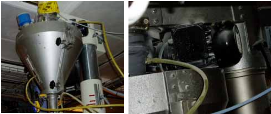
Figure 15.12. The filling funnel, which doses the powder into bags. A rotating 'snail' is fitted to keep the powder 'flowing' and it is driven by a geared motor containing oil. The gear is difficult to inspect.
