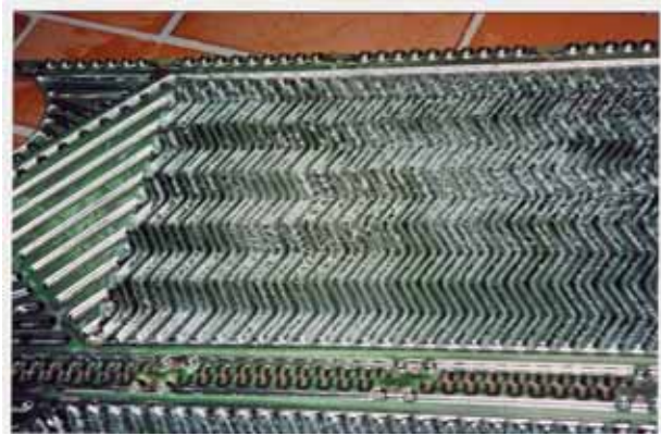
Figure 15.6. A greasy surface with an unpleasant odour from an opened DuoSafe heat exchanger.
