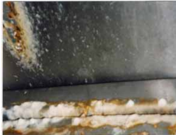
Figure 15.15. A machine producer's idea of hygienic design may be very different from that of a food producer. In this case, it meant that a newly designed machine had to be completely redesigned, costing time and money.
