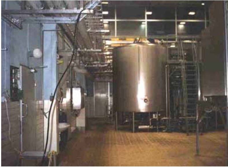
Figure 4.1. Processing area in plant A.
