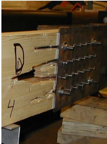
Figure 10. Partial row shear failure, only very few row shear occurred.
