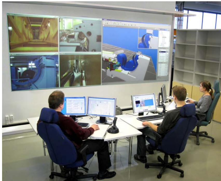
Figure 5.7. DTP2 Supervisory System operating in the Control Room.
