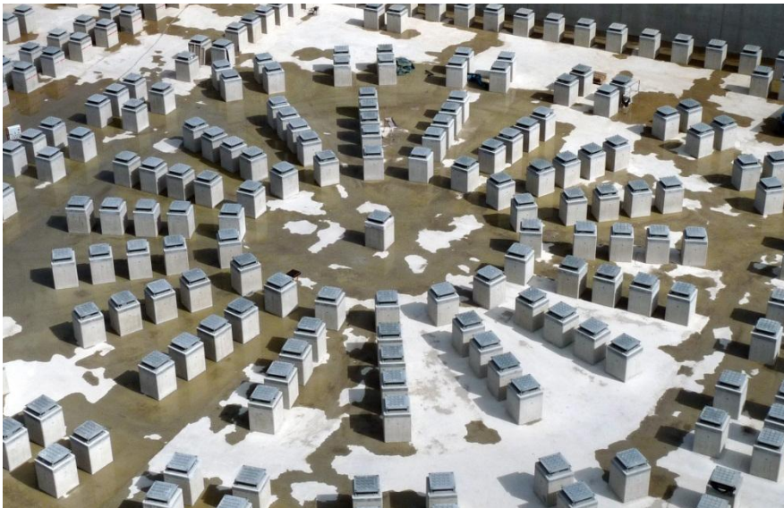
Figure A.3. Seventeen metres below the surface of the platform, the concrete basemat, retaining walls, and seismic pads of the Seismic Isolation Pit are in place to protect the buildings and the equipment from ground motion in the case of an earthquake. Credit © ITER Organization, http://www.iter.org/
