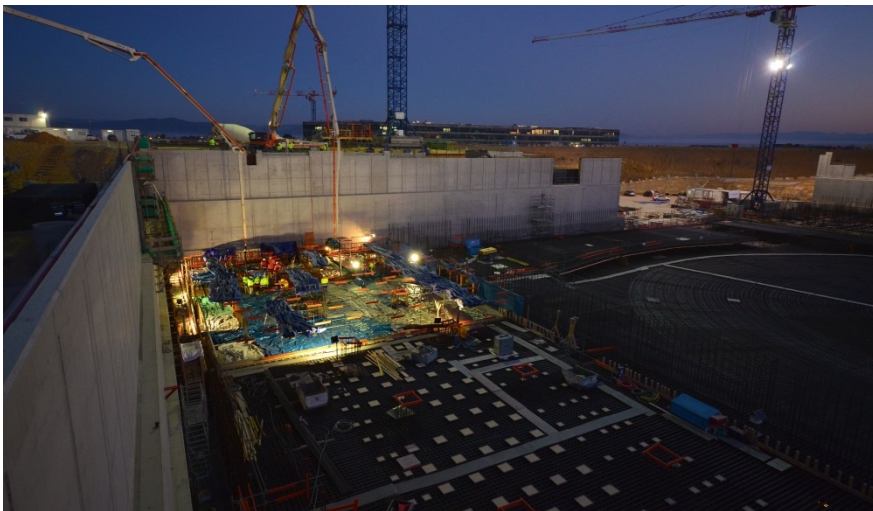
Figure A.3. On the morning of 11 December 2013, concrete pouring begins for the basemat of the Tokamak Complex. Six months, and another 14 “pour days” will be necessary to complete the 1.5-metre-thick slab that will support the weight of the Tokamak, Diagnostic and Tritium buildings. Credit © ITER Organization, http://www.iter.org/
