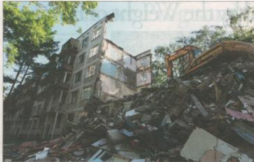
A bulldozer crawling over a pile of debris during the demolition of one of Moscow's five-story apartment blocks.
