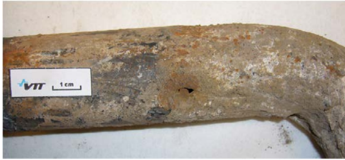
Fig. 3. Photograph of the tube failure, which had caused leakage in the cold economizer of a biomass boiler.
