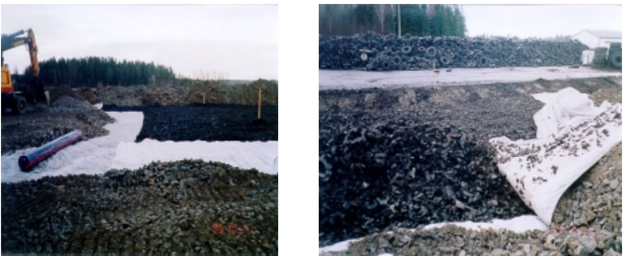
Figure 4. Construction of the upper layers in the RR2 tyre chip area and the bulging of the tyre chip layer due to uneven overload.
