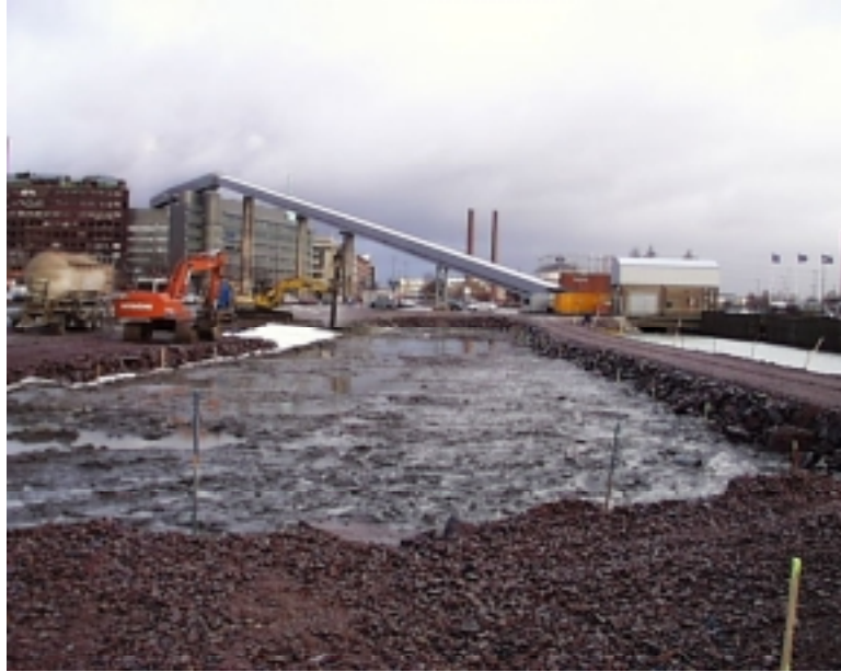
Figure 4. Mass stabilisation work and construction of the compact layer in Sörnäinen, Helsinki.
