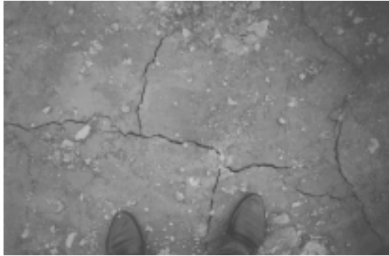
a) Cracks on surface of stabilized clay mass membrane.
