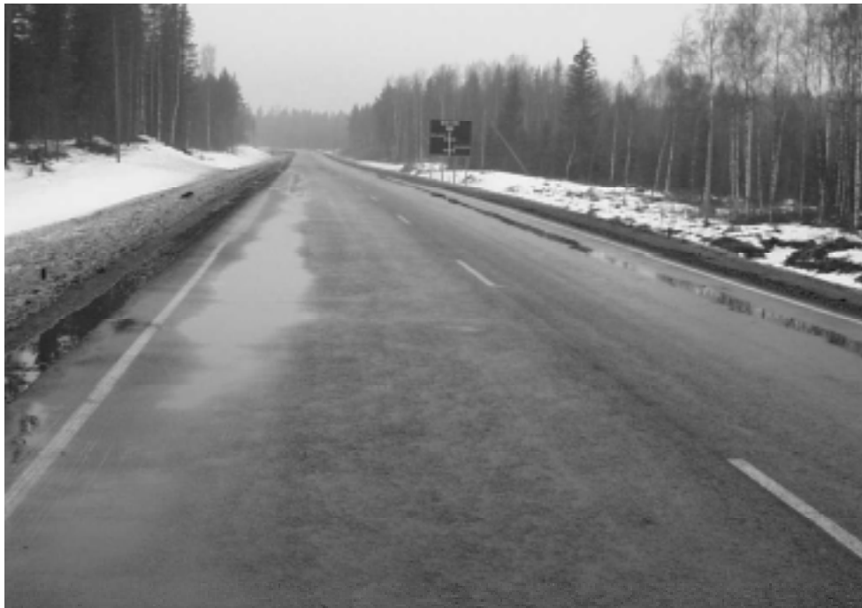
Figure 5. Pooling due to uneven frost heave of fly ash structure in spring 1999.
