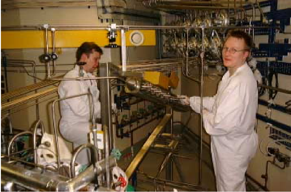
Figure 3. Installation of primary circuit water chemistry and oxide behaviour monitoring cells at the Loviisa plant.
