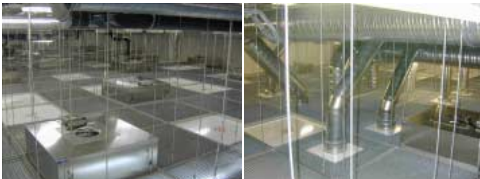
Figure 2. Clean room ceiling & air conditioning system.
