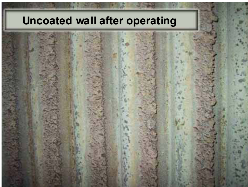
Figure 4. Uncoated wall after operation in “Siekierki” Power Plant.
