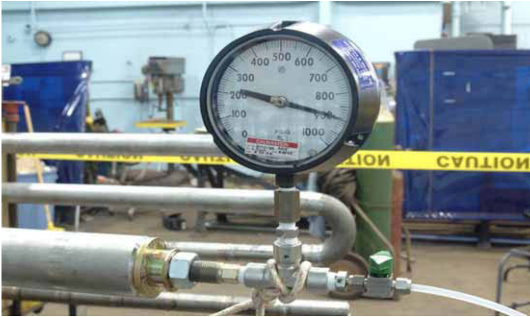
Figure 7. Hydrotesting of Test Loops Prior to Installation in a Boiler (Walt Mohn & Denny McDonald, B&W).
