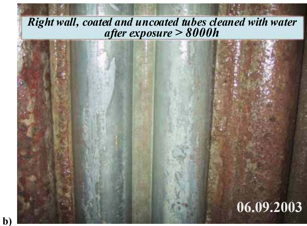
Figure 6. Photographs of the water walls in “Siekierki” Power Plant protected with hybrid coating a) after 4000 h operation, b) after more than 8000 h of operation.
