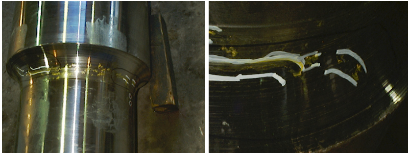
Figure 8. Defects looking like cracks.
