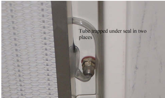
Figure 5.1. Picture showing tube trapped under the filter gasket.
