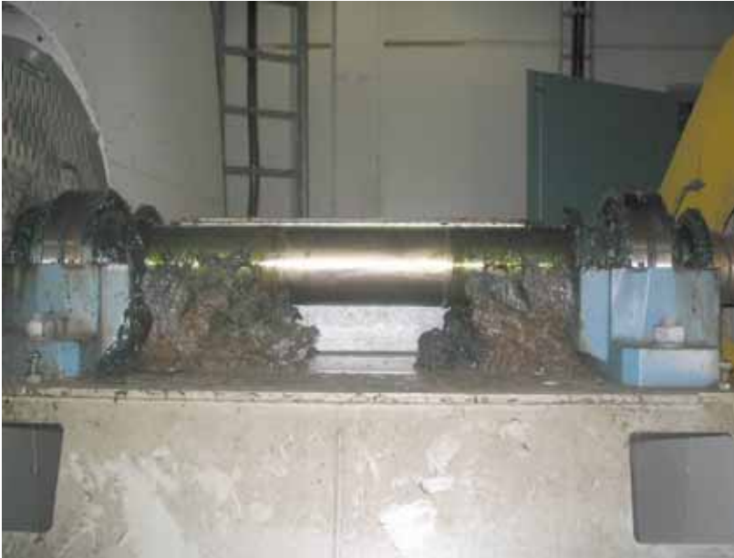
Figure 2. Grease-lubricated bearings at an industrial site (UPM-Kymmene Oyj).
