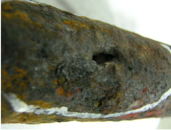
Figure 14. Thick deposits layer near to failure.
