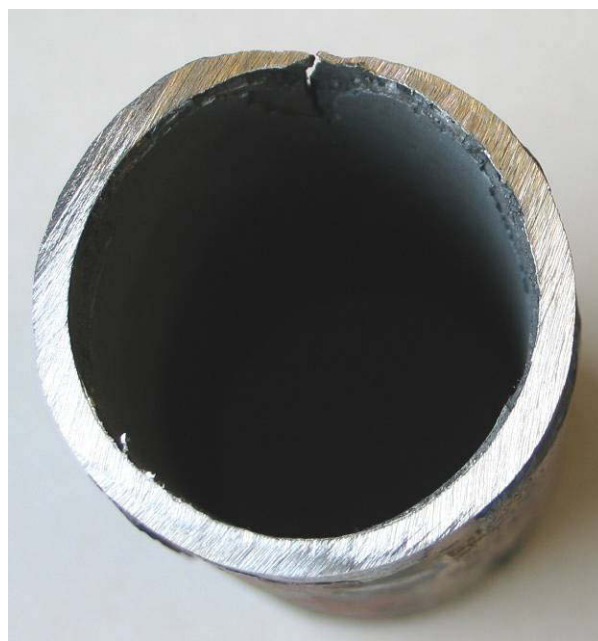
Figure 5. The wall tube thickness loss from the flue gas flow side.
