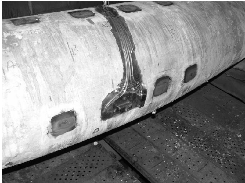
Figure 12. Capacitance strain gauges shown installed on an X20 steam pipe component (24).
