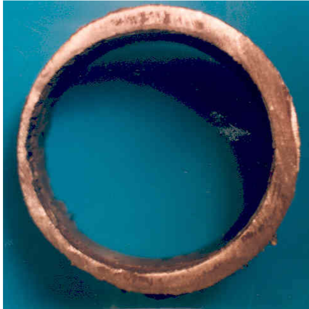
Figure 13. Corrosive wall tube thickness loss on internal surface.
