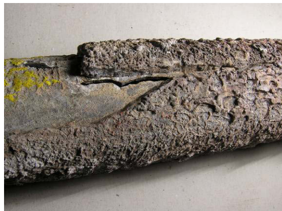
Figure 4. Longitudinal crack, thick layer of deposits on the tube surface.
