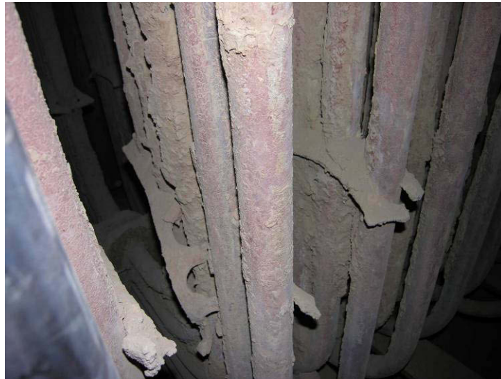
Figure 16. Deposits on external surface of the reheater.
