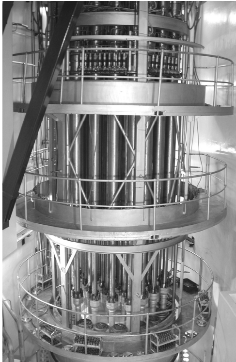
Figure 1. Closure head and control rod housings.
