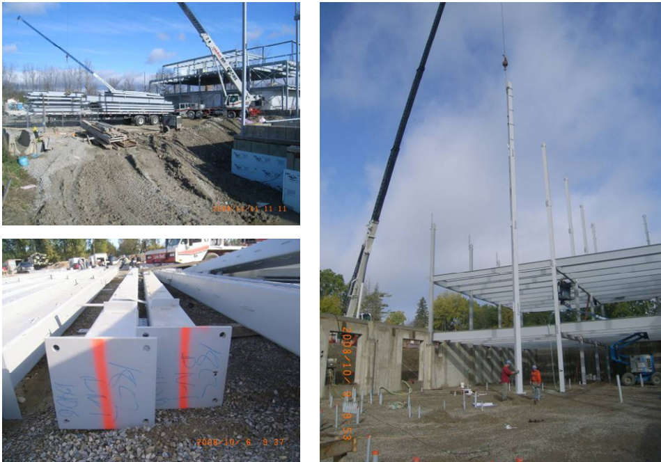
Figure 2. Top left picture shows the steel assemblies received at a construction site on trailers. Bottom left shows the steel columns after unloading and shake out. The right picture shows the erection of a column.
