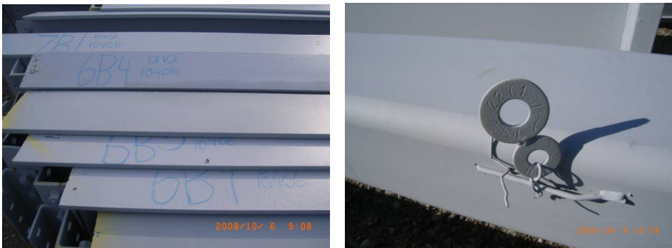
Figure 4. One of the steel beams on the left picture is marked as 6B4 for “DIV 2” erection sequence for the project identified as 10406. The right picture shows a column labeled with a circular disk tag with the identification number 22C1.
