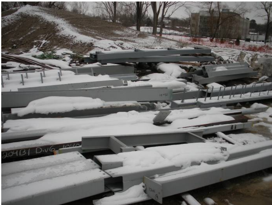
Figure 1. Finding snow covered components could be very frustrating.
