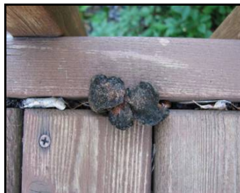
Figure 5. Current above-ground test methods may not adequately account for the accumulation of organic debris that can occur in-service.
