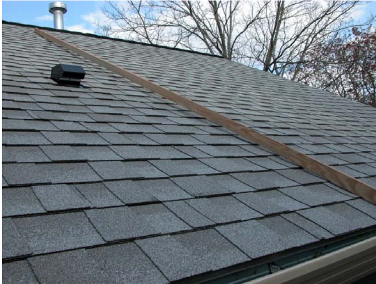
Figure 1. Noticeable sag of rafters on a single-story home of modest size, constructed in 1940. At the time of construction, regional building codes had not been developed.
