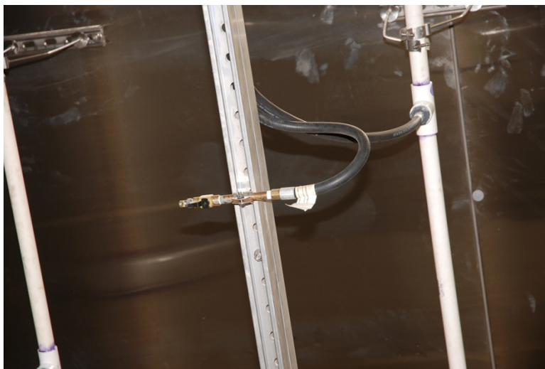
Figure 3. One of 16 spray nozzles mounted near the chamber ceiling.
