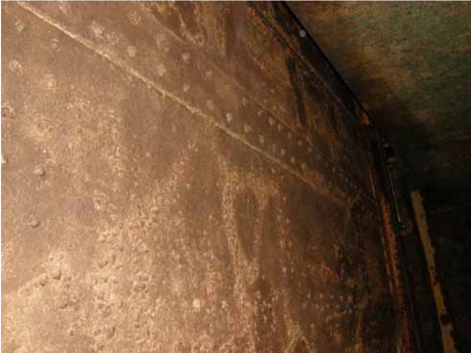
Figure 1. Deterioration of a steel cover plate of quick-closing valves.
