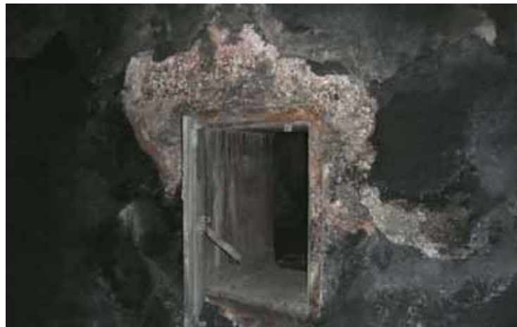
Figure 5. Post-fire inside appearance of the bottom maintenance door opening [1].
