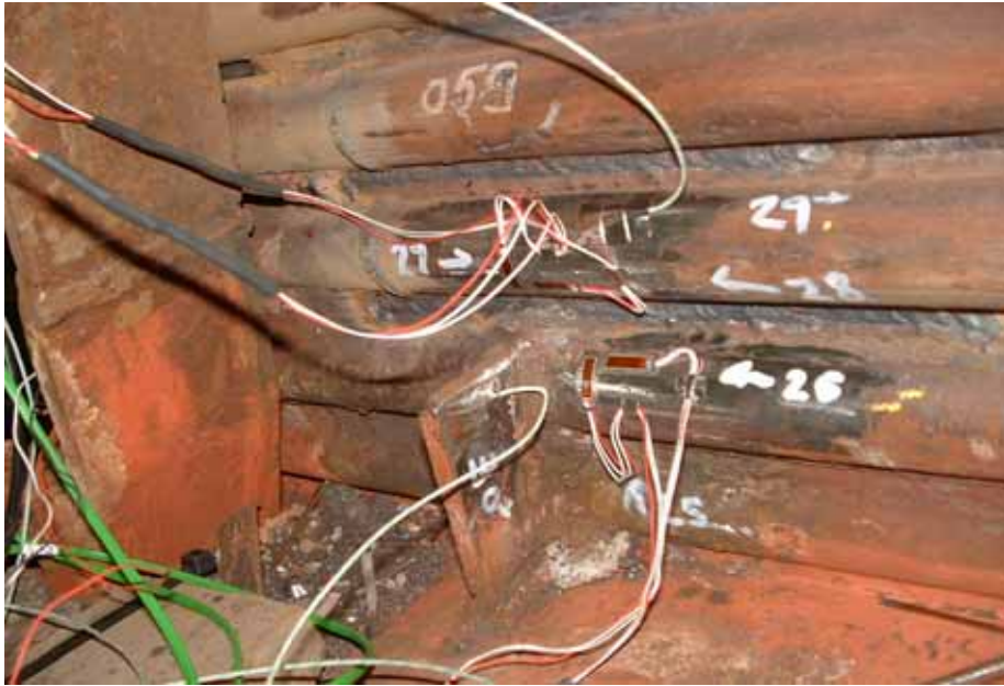
Figure 7. Typical strain gauge installation.
