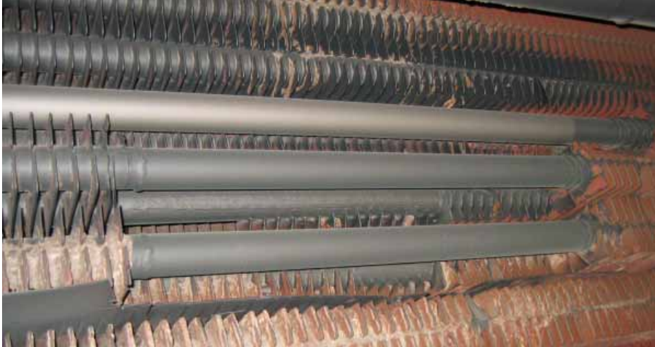
Figure 2. A coated tube installed into an economiser in boiler 2.
