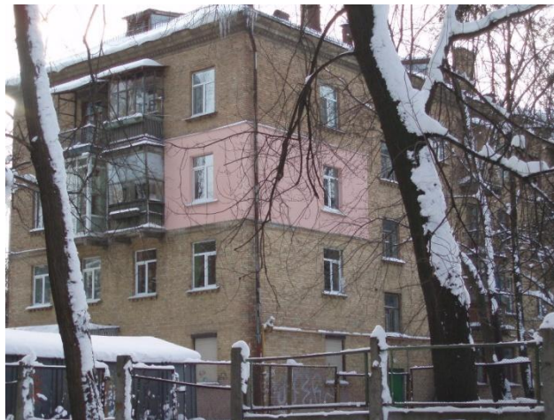
Figure 133: home alone – one apartment externally insulated and rendered. (Photo credit: Andres Järvan).
