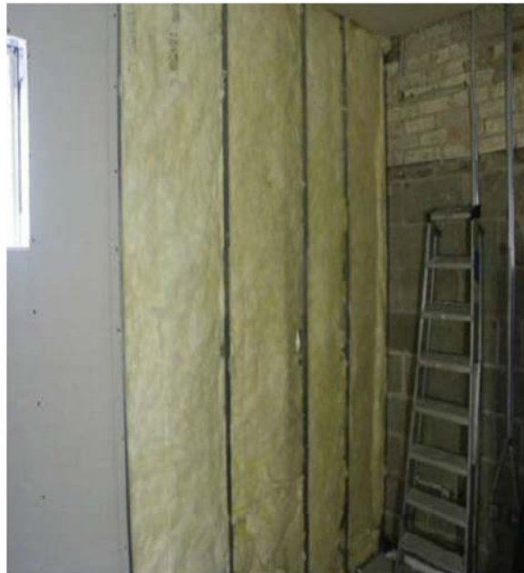
Figure 12. Installation of freestanding steel studwork internal insulation with an air cavity. (EST2005)
