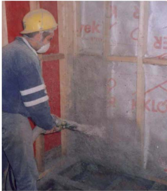
Figure 13. Installation of freestanding wood studwork internal insulation with an air cavity. (EST2005)
