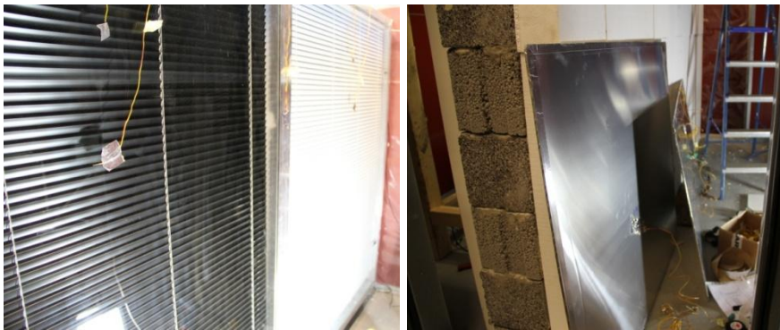
Figure 4. Blinds installed behind the glass façade (left) and PCM-panels at the building phase of the wall (right).
