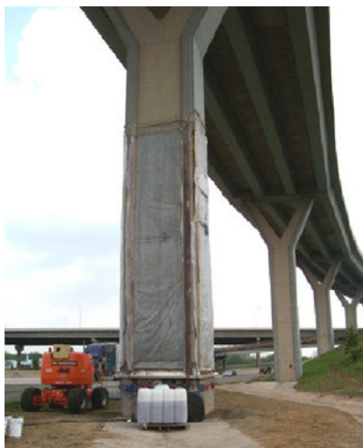
Figure 4. The field application of the electrochemical lithium treatment in a bridge in USA (Bentivegna et al. 2011).
