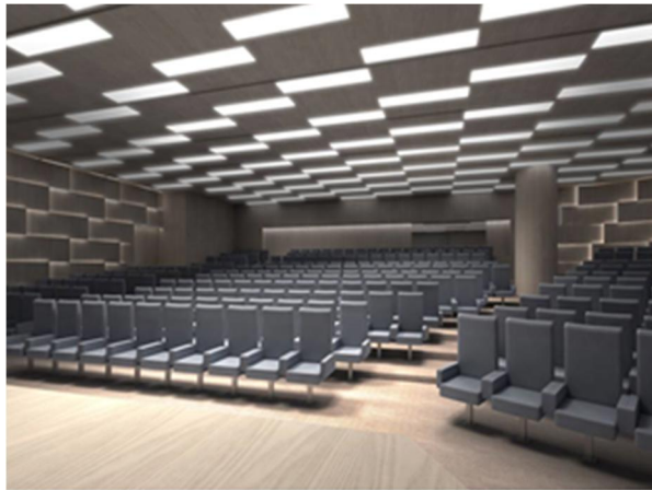
Figure 74. The lights in the auditorium are operated with an intelligent control system (Zhou 2012).
