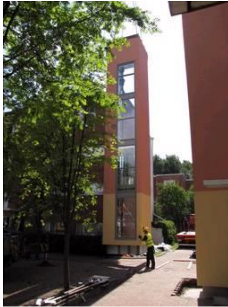
Figure 61. In the Lehdokkipolku 3 housing cooperative in Helsinki, NEAPO adopted a new approach of installing elevator cars and machinery inside the lift shaft while this was still in the factory (NEAPO 2009). Thanks to factory-installation, the lifts became available for residential use too.
