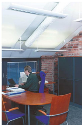
Figure 79. The Sensus® panels provide the heating, cooling and indirect lighting to the offices in Blomstedt Hall. (Photo: ARE Oy.)
