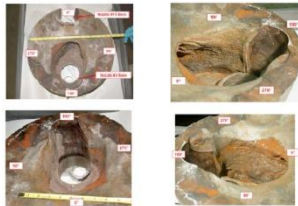
Figure 5. Davis Besse RPV penetration.
