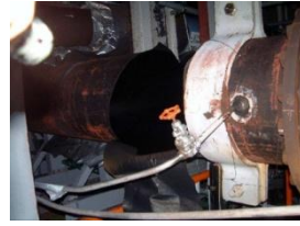
Figure 6. MIHAMA Flow Accelerated Corrosion.
